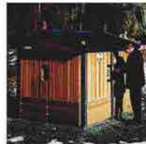
紧凑型二次变电站 Compact distribution substation
